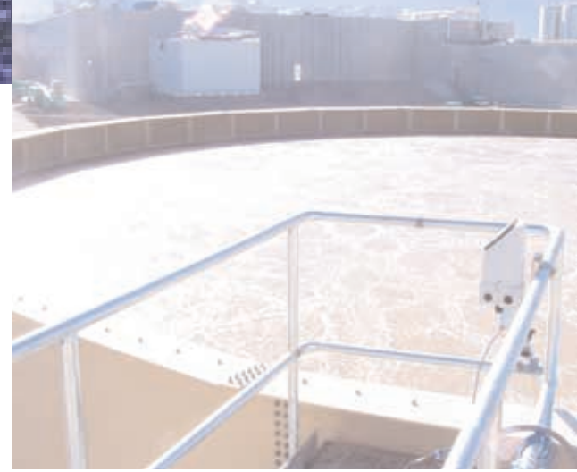
Disc diffusers in operation.
