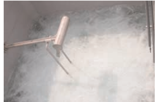
Tube diffusers in operation
